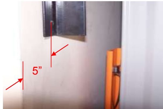
Figure 15. Jamb Stop and Exit Hardware
